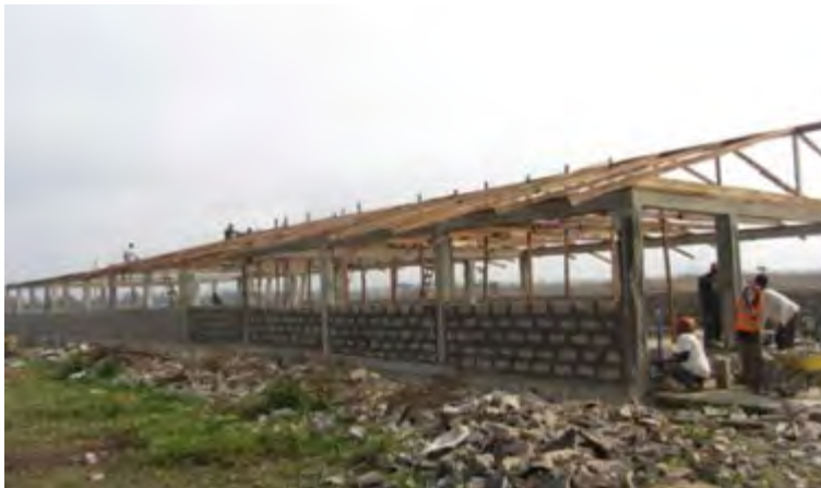
Figure 13: The ongoing construction of the livestock quarantine facility at CARI, in Bong county.
