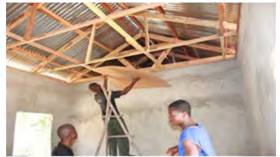
Construction workers begin the ceiling work of the rice processing center in Doumpa, Nimba county.
