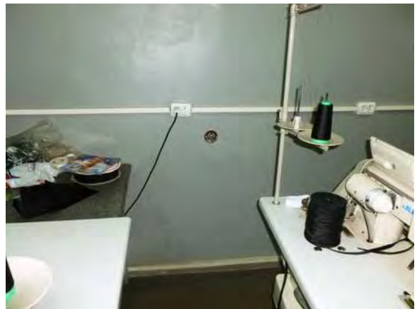
Unsafe power socket.
