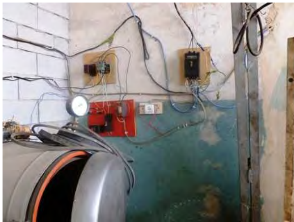
Factory electrical wiring.
