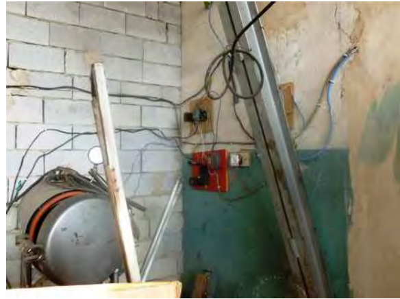
Factory electrical wiring.
