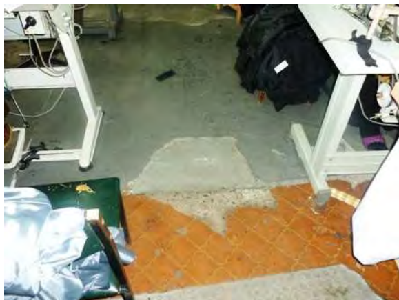
Factory floor is damaged.
