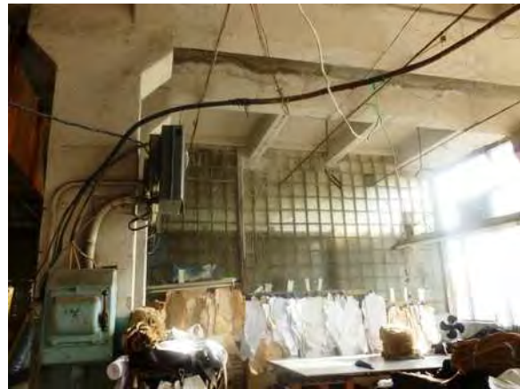
Factory electrical wiring.
