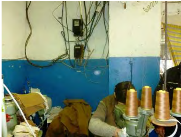
Factory electrical wiring.
