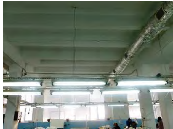
Smoke detectors and ventilation system.
