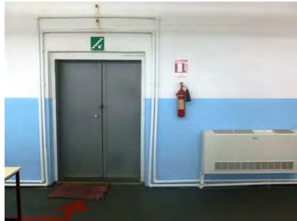
Evacuation door is not properly installed.
